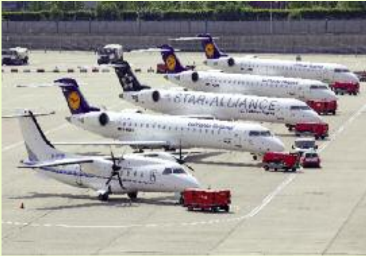
Diesel generators (Ground Power Units) supply electricity to aircraft at remote positions.
