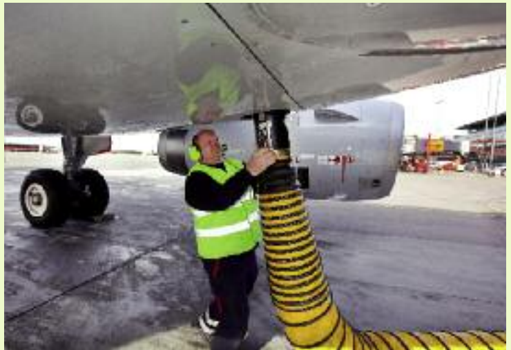
At Pier parking positions, the aircraft are supplied with electricity and air conditioning from the block-type thermal power plant.
