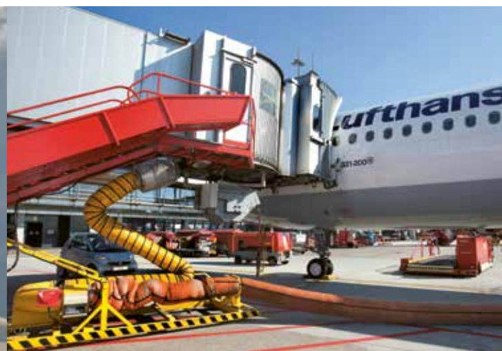
At Pier parking positions, the aircraft are supplied with electricity and air conditioning from the block-type thermal power plant and the APU remains switched off
